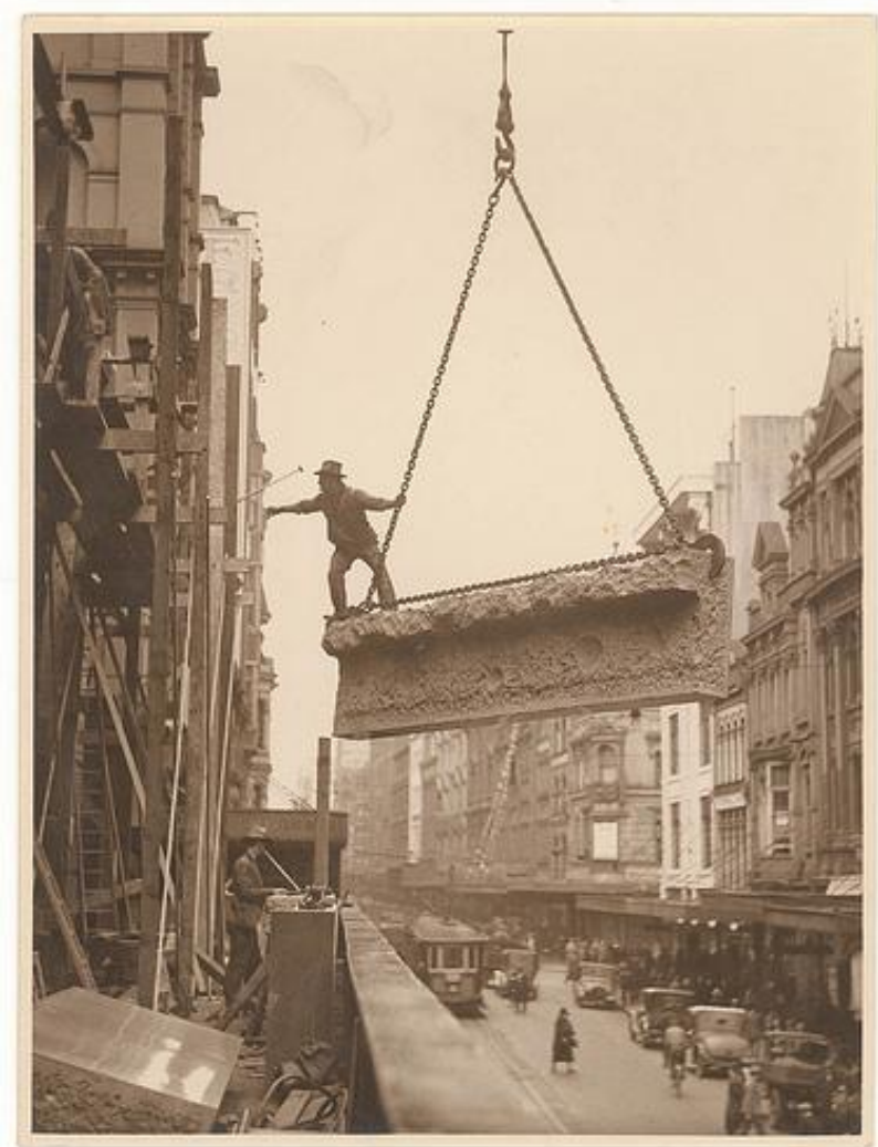
Building labourer on a stone being hoisted up to building, Pitt St, Sydney, c. 1930s, by Sam Hood No known copyright restrictions.
